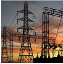
CRITICAL POWER SUPPLY
